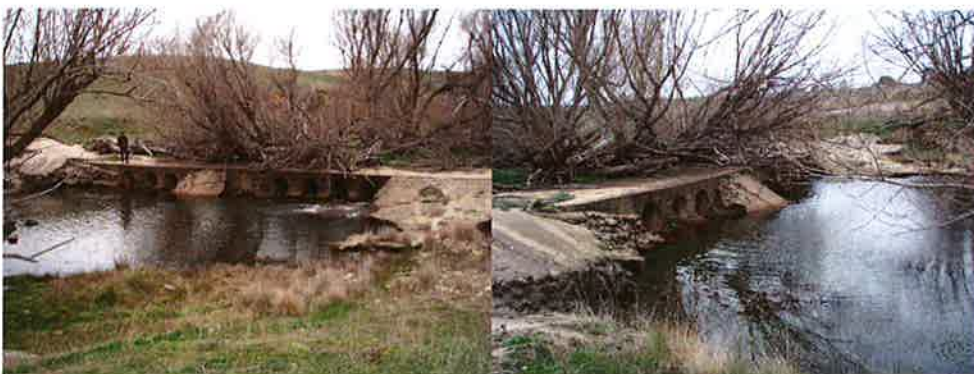
Figure 8: Disused road crossing on the Bolong River (at Lat 34.29718, Long 149.62540)
