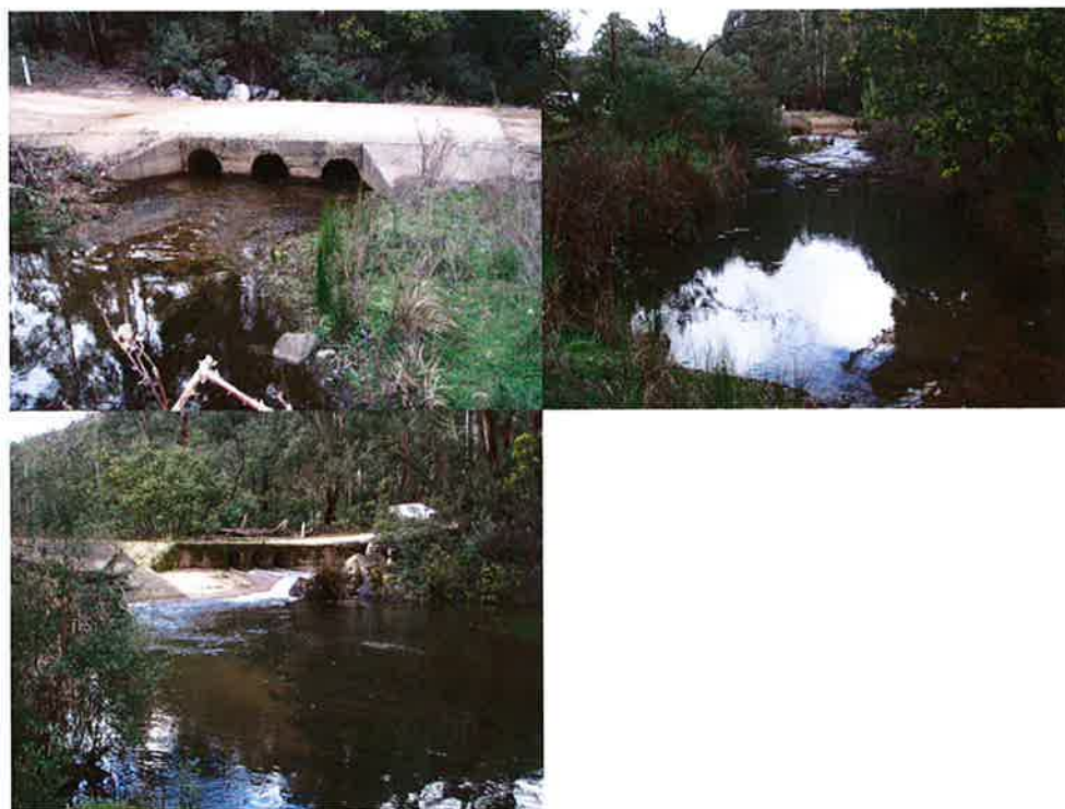
Figure 12: Road crossing forming a fish passage barrier on the Mt Werong Creek (at Lat 34.1657, Long 149.8756)
